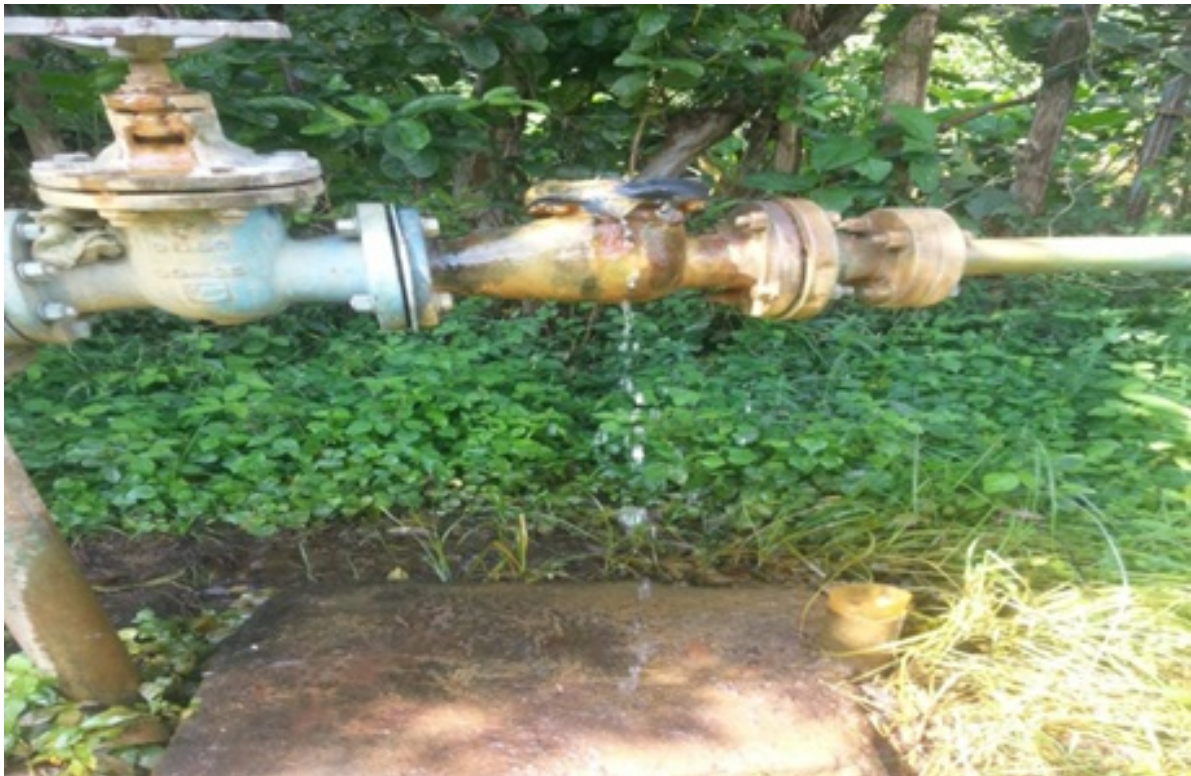
Figure 3 Typical Borehole as Water Source of Dilla Town
